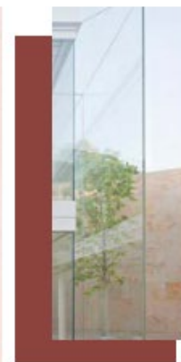
D- Window frame Rusty red colour steel window frame
